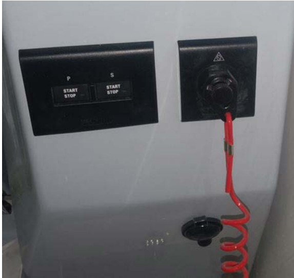
Engine Stop Switch
