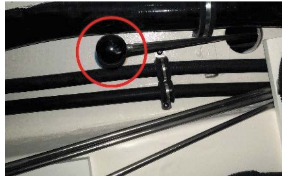
Deck drain ball valve levers
