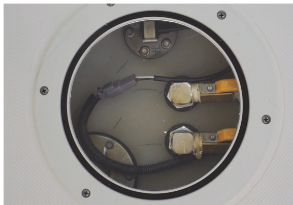
Gas Tank Valves
